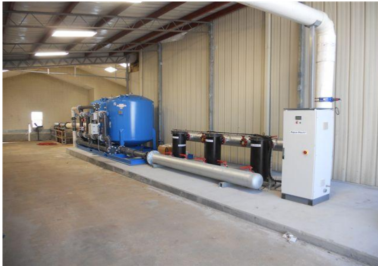
The main water room at Metrolina Greenhouses
